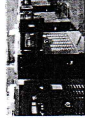
South Sudan - Juba MPMC product: 7 units of 17kva Kubota silent generator sets Key words: MPMC Customized options: special color powder coating, residential muffler
